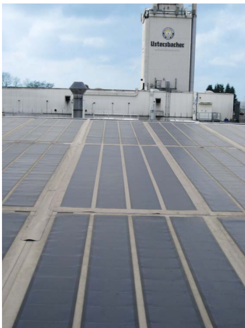
Ustersbacher Brewery, Ustersbach, Germany, 65 kWp
