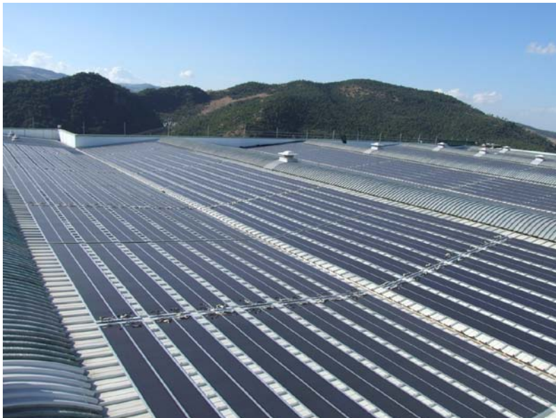
One of four sites of the Coca-Cola Hellenic Bottling Company, Monticchio, Italy 472 kWp of total 3.3 MWp
