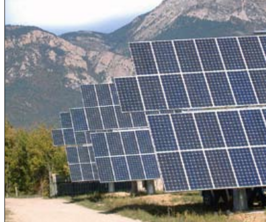
Polar tracker by the Spanish company Feina: Polar trackers should be installed in such a way as to not cast shadows on each other.
